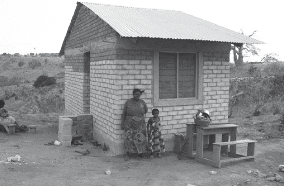
A core house (phase one of a bigger house) built by a member of Makazi Bora group with technical assistance from WAT. Photo taken by WAT.
