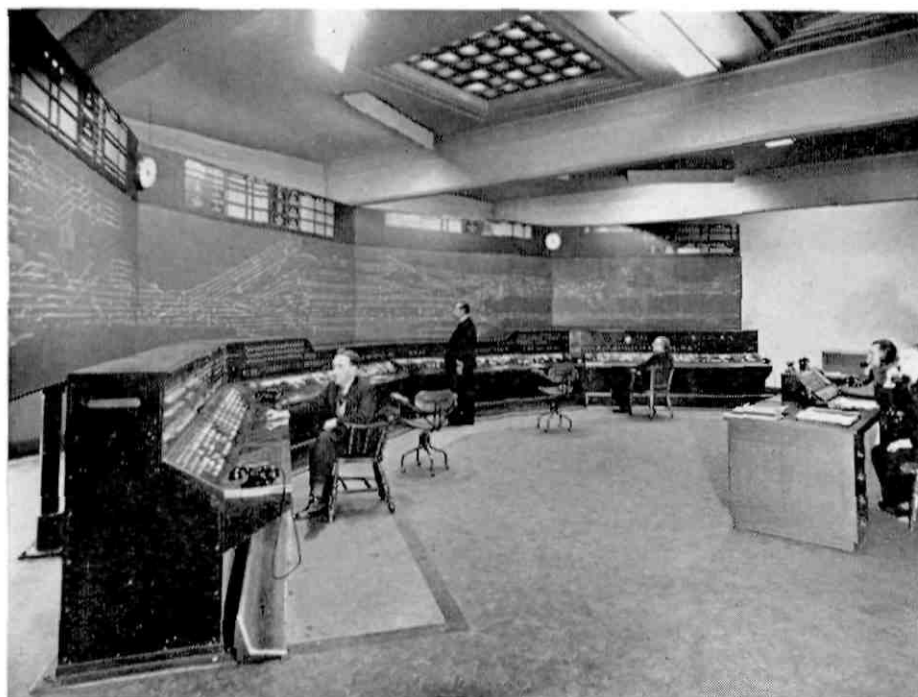
First stop on the group's rail journey through Britain was at York, where they inspected the huge central control room of the York signalbox. This controls 33¼ miles of track in and around the city of York, one of the towns the party visited (Photograph by courtesy British Railways)
