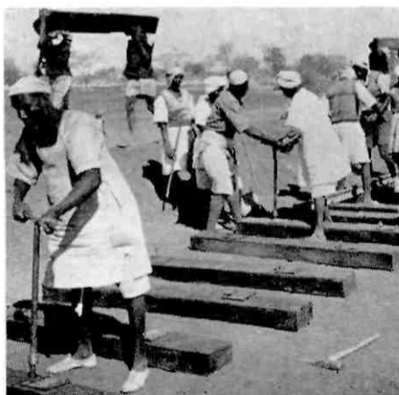
The Sudan Railways are to be extended under the new seven-year plan. This photo shows work already in progress on the construction of a new railroad from Sennar Junction to Singa in the Fung area - a total length of 66 kilometres (Photo: Sudan Government Public Relations Office)
