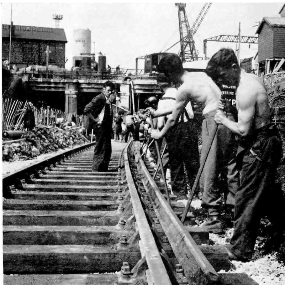
The future pattern of track maintenance will be a mobile maintenance gang, fully mechanized, centred in towns and cities, probably ten men to cover 20-30 miles of railway.
