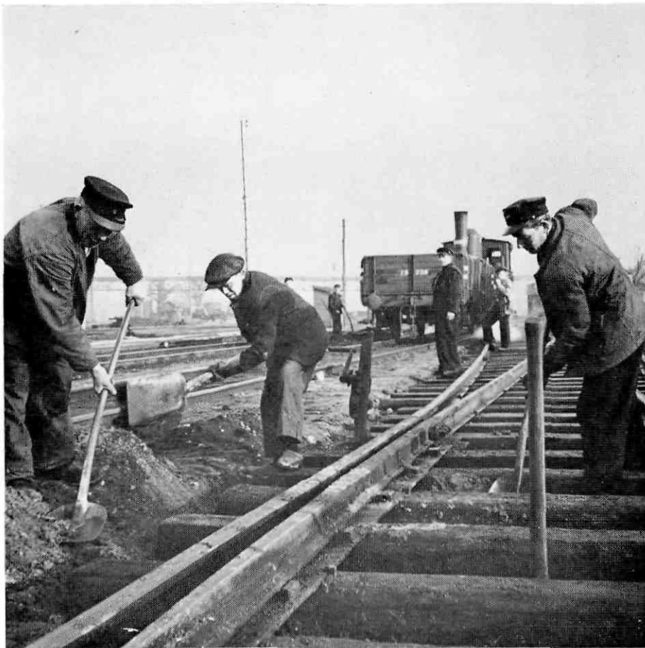
Permanent way workers repair the line; State Railways staff are organized in five unions.
