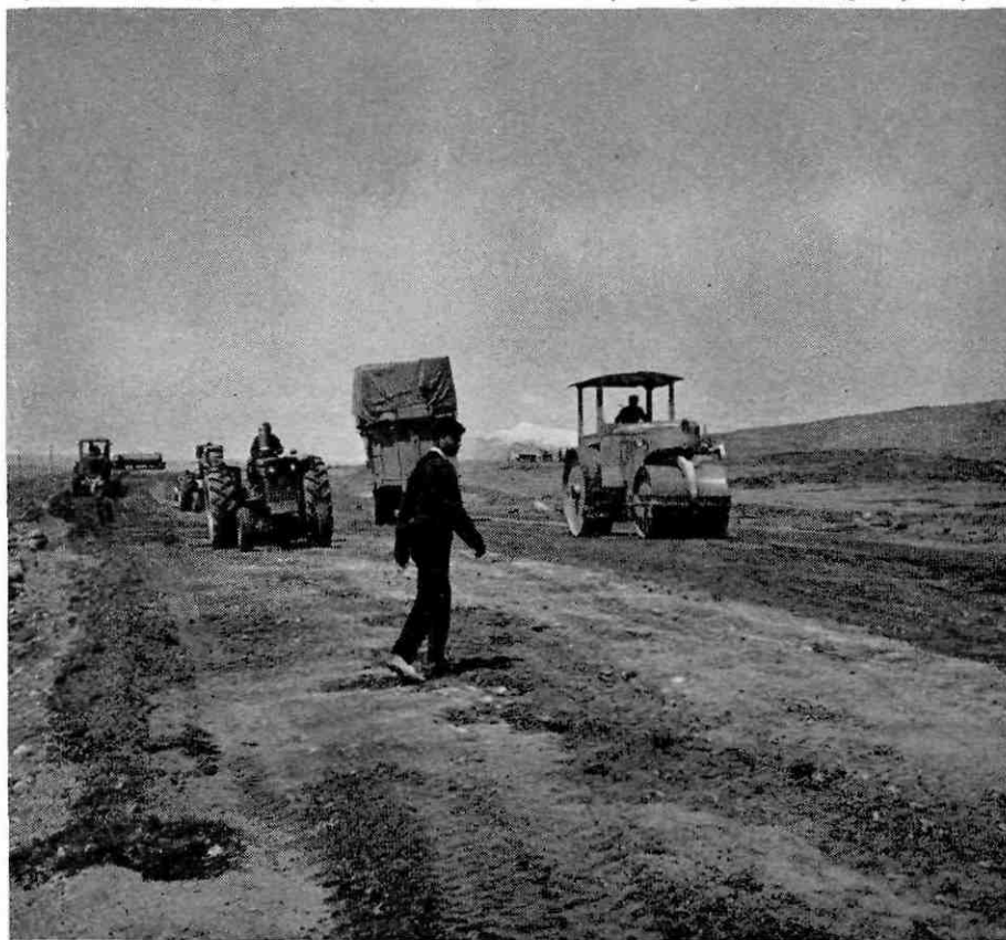
This part of the A1 route is between Tabriz in Iran and the Turkish border. Mechanized equipment is being used to prepare the foundation for a good, hard highway surface.
