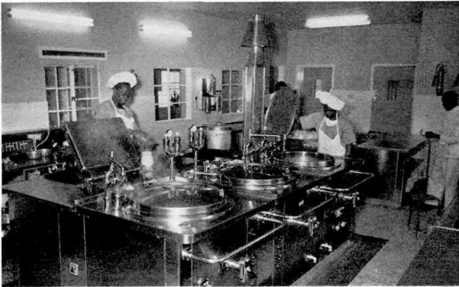
The kitchens at Kampala. The magnificent equipment was given by German unions.
