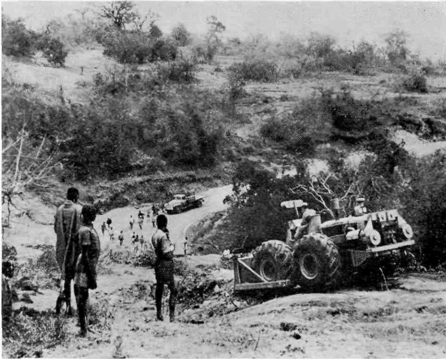
Since 1951 most of the roads in Ethiopia have been renovated. The Italians during their occupation built some 3,000 miles of highway which however were neglected during the years that followed their departure. A road renovation programme was launched in 1951
