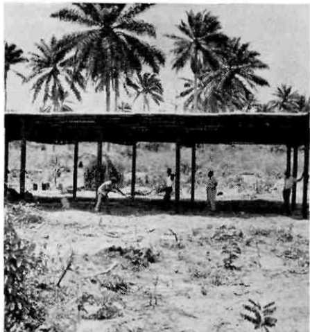
A private contractor levelled out the land for the Motor Drivers' school site free of charge. Work has now been started on the building itself. It will house a workshop (on the far left), classrooms (in centre) and an office to replace the temporary quarters
