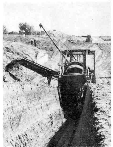
The tractor ditcher shown here can dig up 3,000 feet of clean ditch a day for a pipeline. The ITF has recently adopted a statement of principles concerning the construction and operation of pipelines designed to safeguard workers in the 'traditional' transport industries from unnecessary hardship
