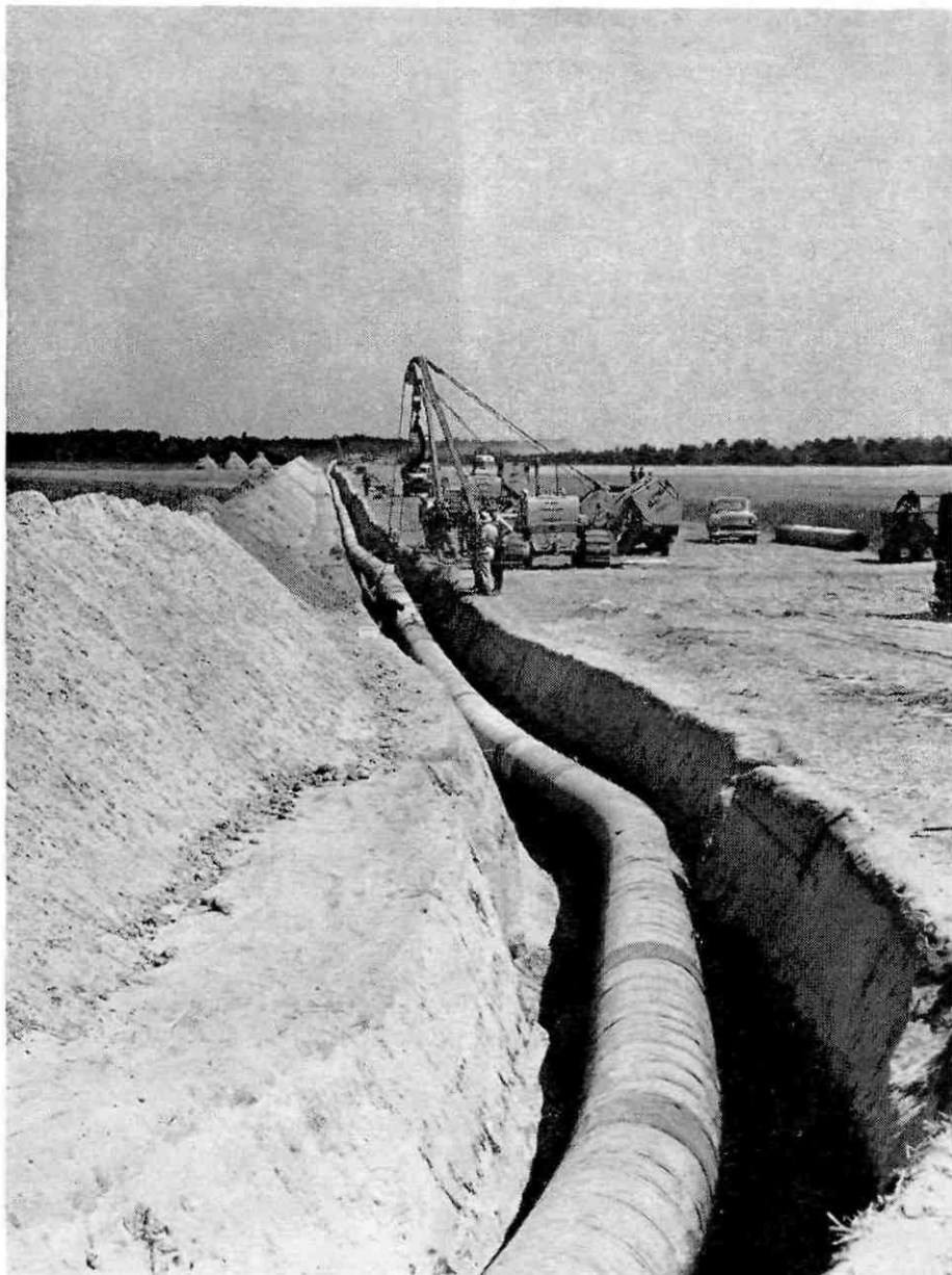
This picture shows a section of the Rotterdam-Rhine pipeline under construction near Venlo in the Netherlands. This 180 mile long, 24 inch line built to take crude oil from Rotterdam to refineries in the Ruhr and Rhineland, together with the Wilhelmshaven-Ruhr line is expected in time to bring an increase in oil traffic to the North Sea ports (SHELL photograph)
