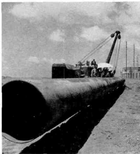
The Iraq Petroleum Company's pipeline, running from the oilfields of Northern Iraq to Baniyas on the Syrian coast, was completed in 1952. This 30 inch diameter line provides overland transport for the IPC's oil where tanker transport could not be used as an alternative: an instance of co-ordination rather than competition in oil transportation (SHELL photograph)
