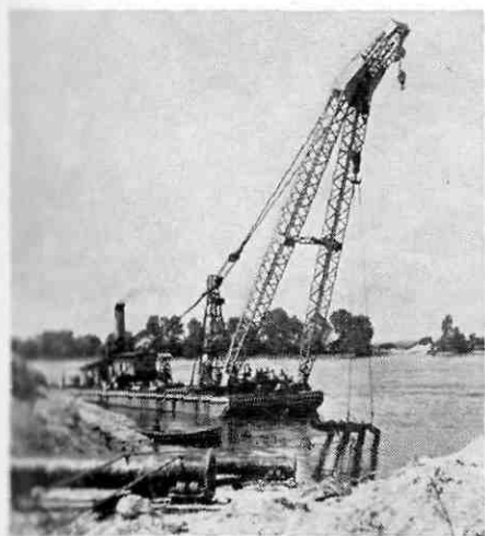
Laying the Le Havre-Paris pipe-line across the Seine at Aiziers. Pipe-lines have certain advantages over the conventional means of transport with which, in a number of cases, they are, or will be, in direct competition
