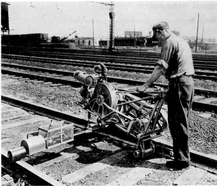
Maintenance-of-way crews can cover greater distances than was ever previously possible by using modern machines such as this new one-man power wrench (Nordberg Manufacturing Corp.)
