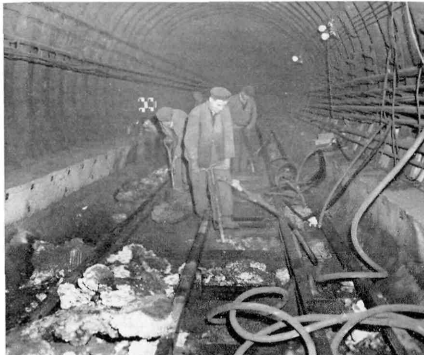
Permanent-way workers breaking up the concrete bed of the tunnel. One of the many jobs going on whilst London's ten millions are fast asleep in their beds. Essential jobs of repair, cleaning and maintenance have to be done at night during the period of five hours or so when the current is switched off and no trains are running (Photograph by LTE)
